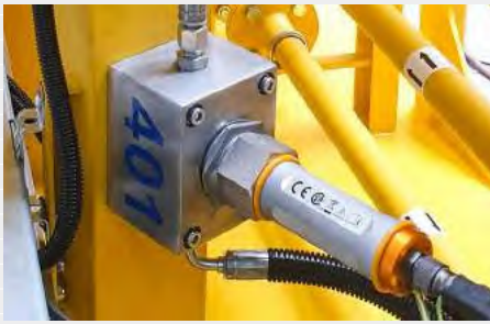
MicaSonic™ applied on a VOP plant to measure - Breakdown voltage [kV] - Moisture content [ppm] (@ 20°C and actual temperature as per IEC)
